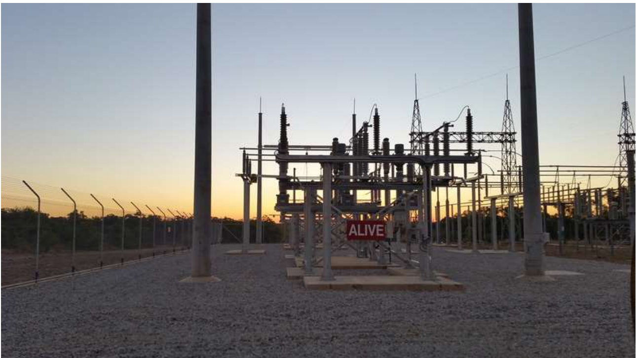
Figure 5: Cut-over works successfully completed for the 132kV line into the Ergon-Kidston substation.
