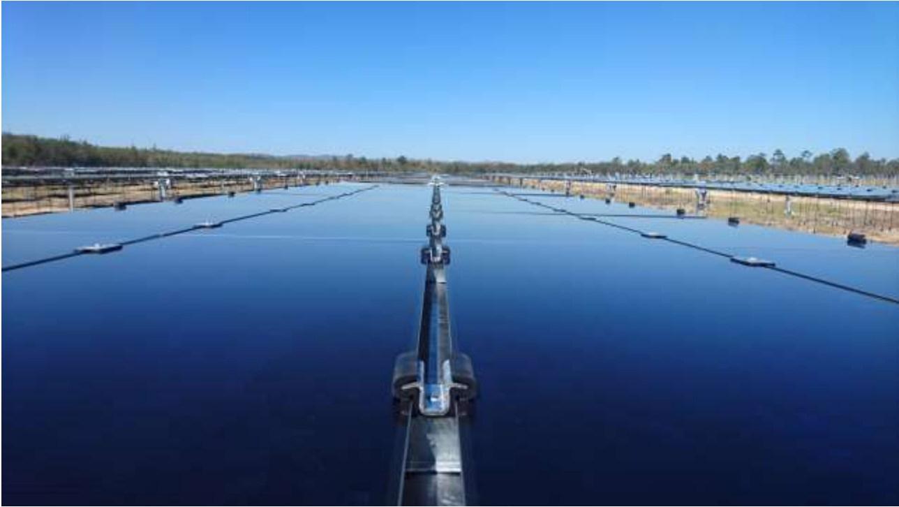
Figure 3: First-Solar Inc. thin-film modules expanded across the site.
