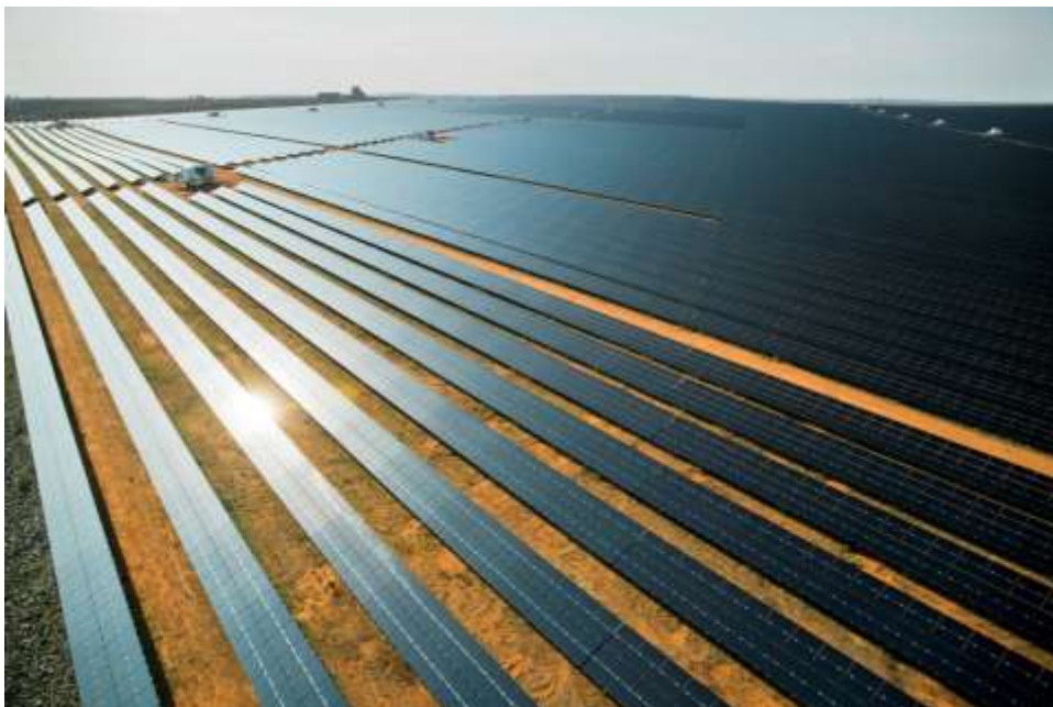
Figure 1: First Solar, Inc. PV Modules in use at AGL's Broken Hill Solar Plant – photo courtesy of AGL Energy
