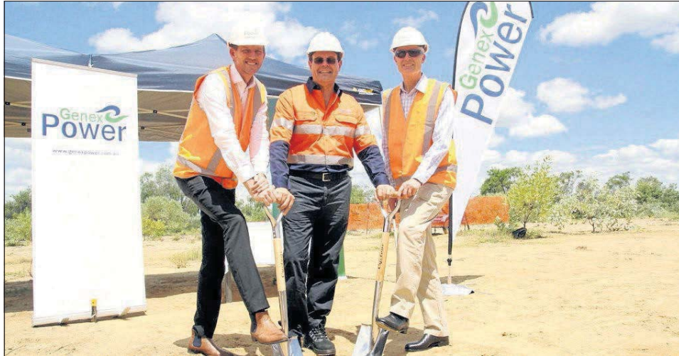
Energy Minister Mark Bailey, Genex chairman Dr Ralph Craven and ARENA CEO Ivor Frischknecht break the soil to celebrate the start of construction.
